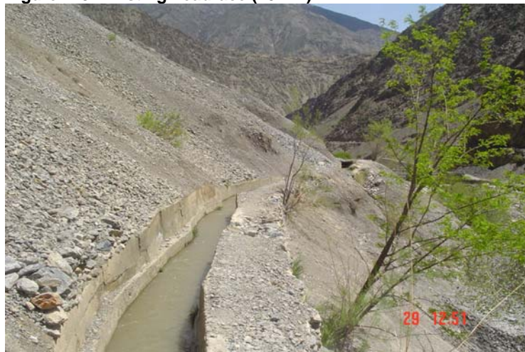
Figure D-5: Existing headrace (40 kW)
