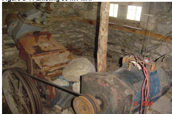
Figure D-7: Existing 50 kW MHP
